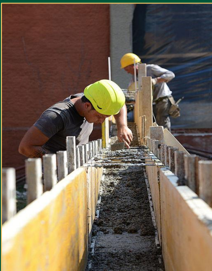
Construction workers place concrete for a ramp (Source: U.S. Army Corps of Engineers)
