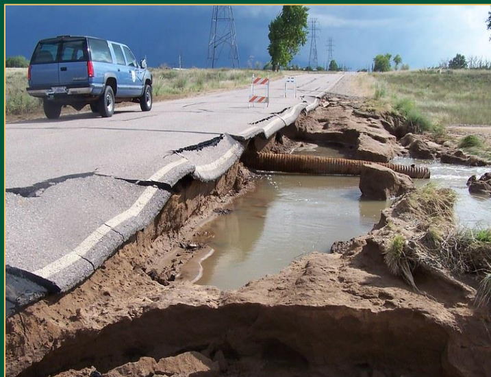
Road damage due to a dam breach in Colorado (Source: USFWS Mountain-Prairie)
